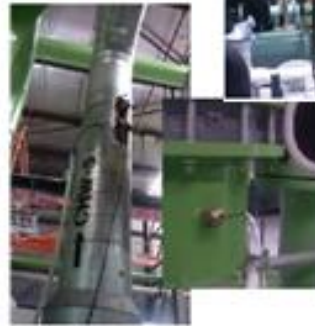
Chilled Water, Condenser Water Temperature & flow rate sensors
