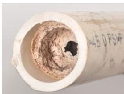
Scale build-up without a Superior Water Conditioner
