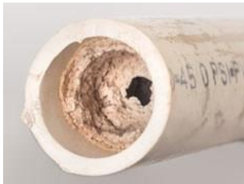
Scale build-up without a Superior Water Conditioner
