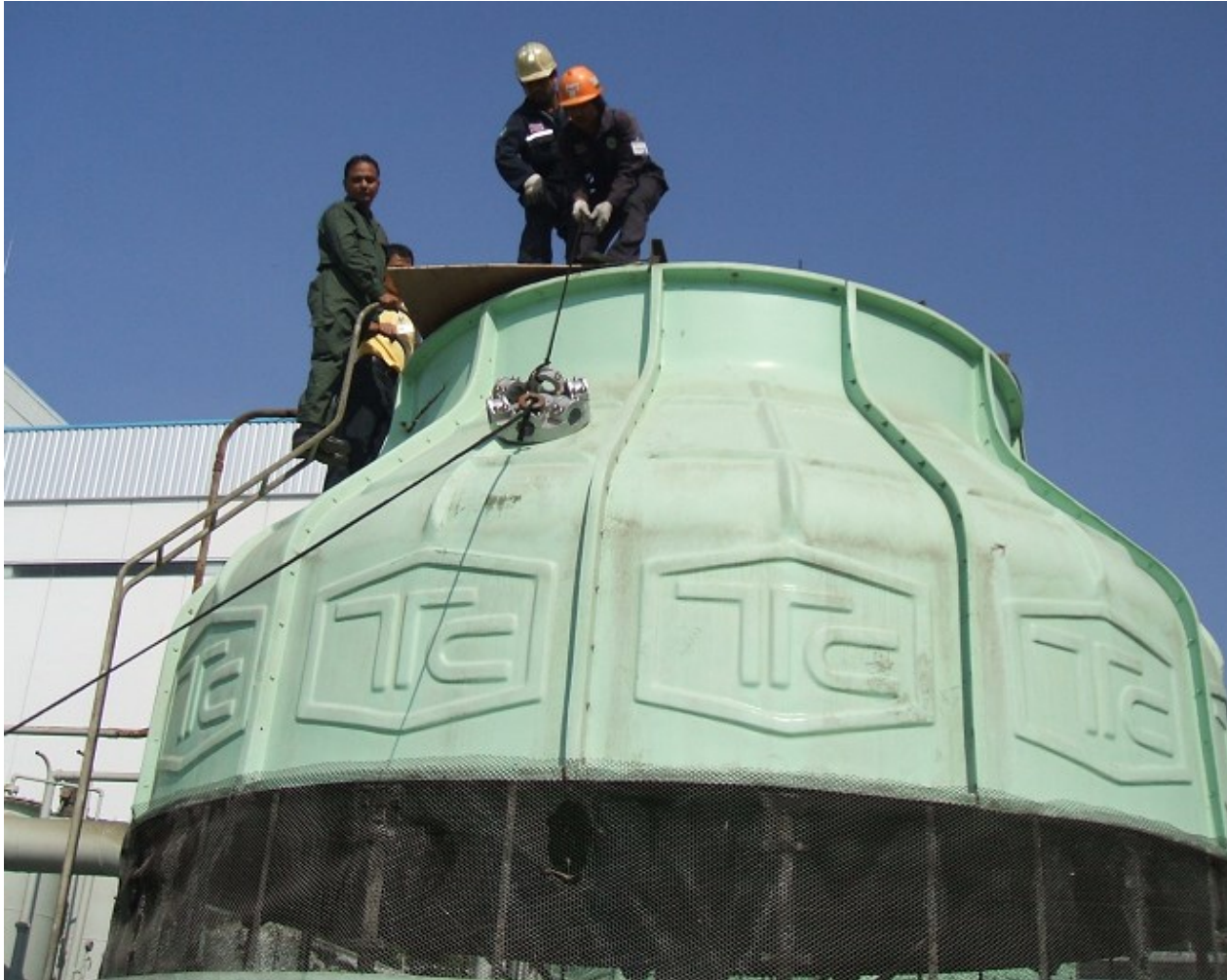
ENCON Hub Installed
