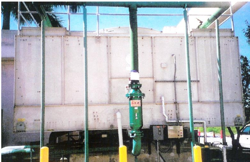
ACV-6-K-10 Installed on a 700 ton Cooling Tower
