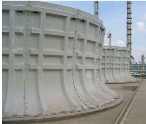
PTTCH Cooling Tower Fan dia. 24 feet
