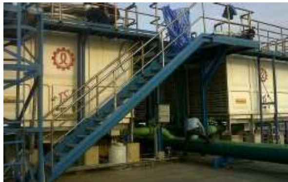
P & G Cooling Tower Fan dia. 2000 mm.
