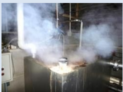
Steam leaking from recovery Tank
