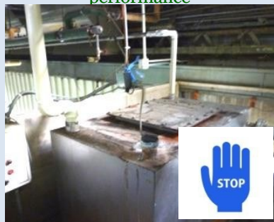
Stop of steam leaking
