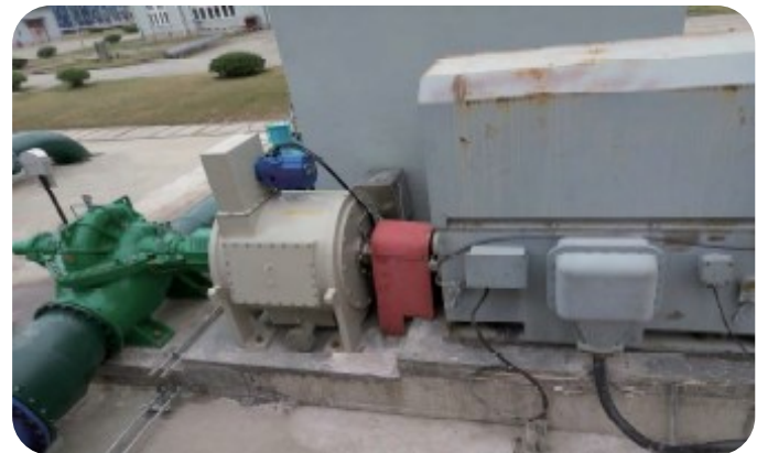
Cooling water system (Petrochemical) 800 kw pump
