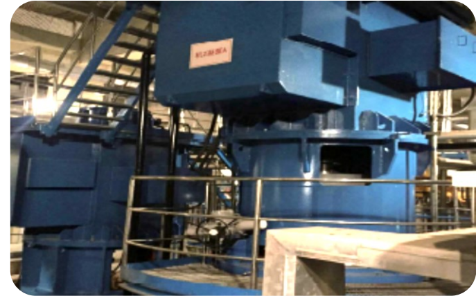
Condensation system (Power plant) 800 kw pump
