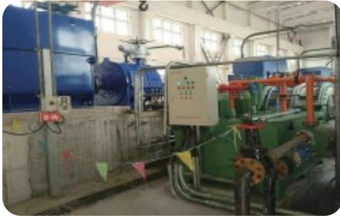
Refinery water system (Petrochemical plant) 800 kw pump
