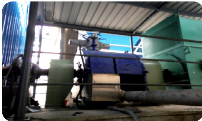
Fan system (Power plant) 1400 kw pump
