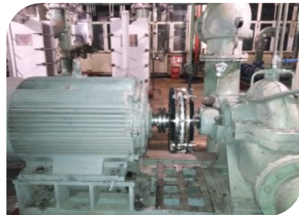
Boiler water system (Cement plant) 155 kw pump
