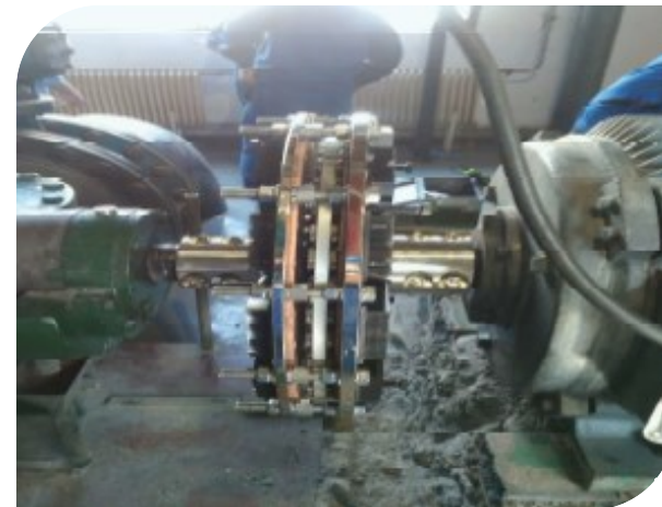
Closed Cooling water system (Power plant) 110 kw pump
