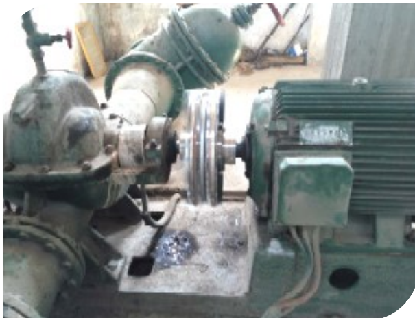
Cooling water system (Chemical plant) 90 kw pump
