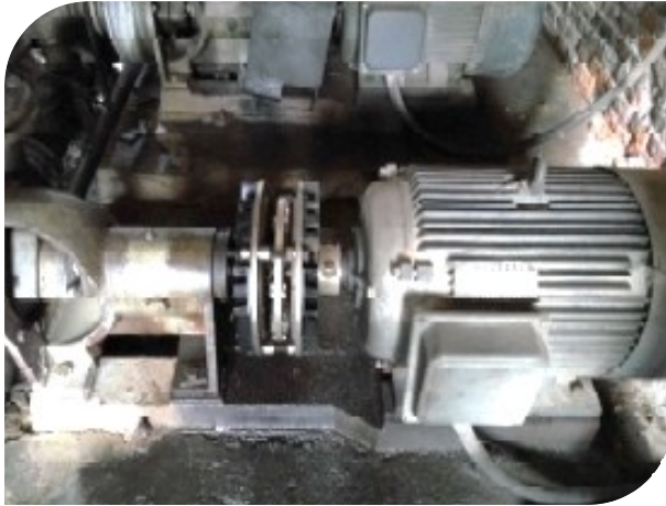
Process water system (Chemical plant) 37 kw pump
