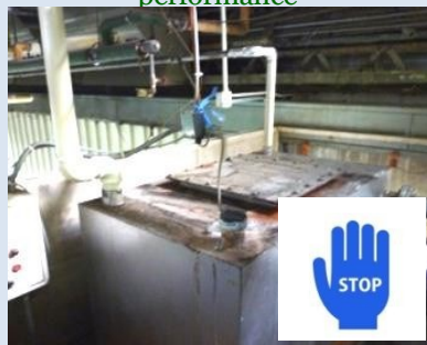
Stop of steam leaking
