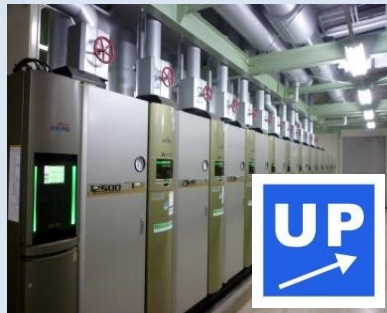
Improvement of Boiler's performance
