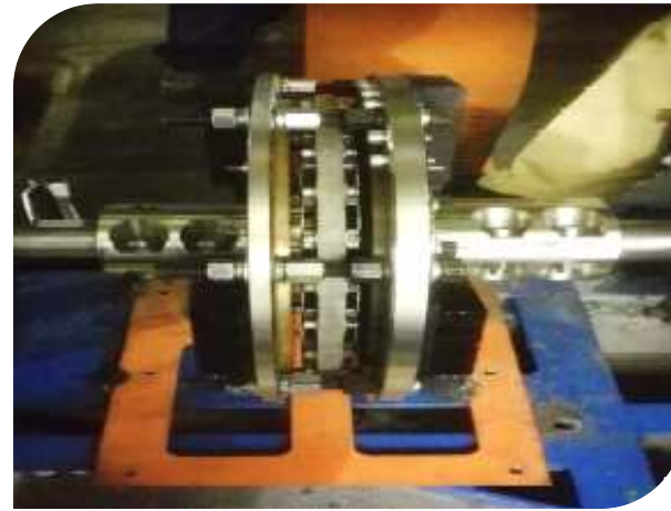
Closed Cooling water system (Power plant) 132 kw pump
