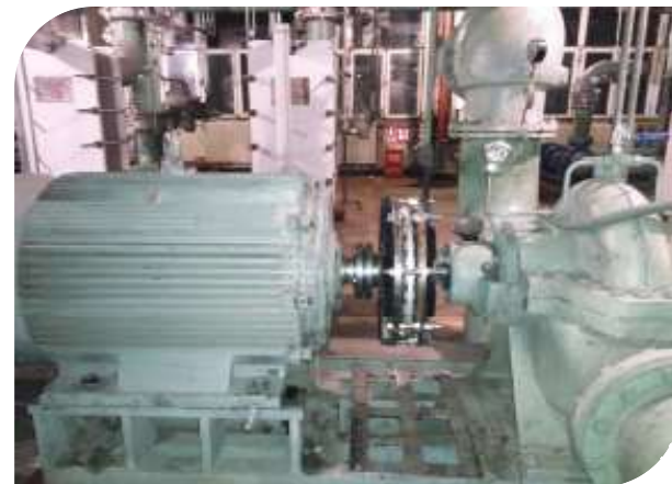
Boiler water system (Cement plant) 155 kw pump
