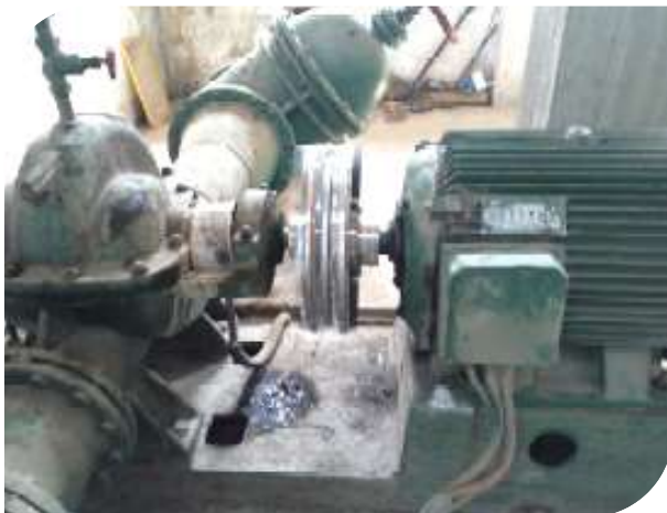
Cooling water system (Chemical plant) 90 kw pump
