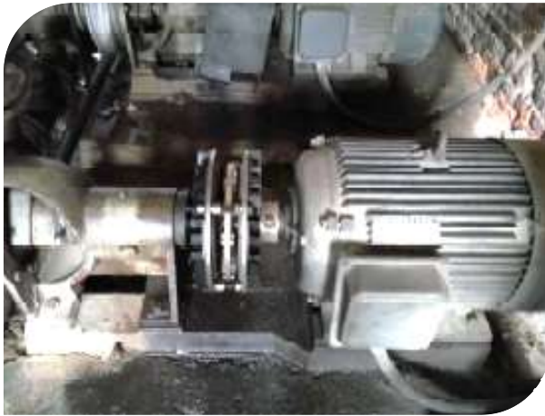
Process water system (Chemical plant) 37 kw pump
