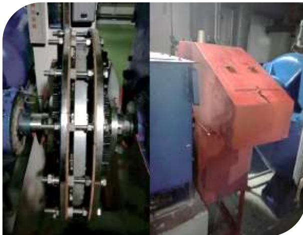
Closed Cooling water system (Power plant) 355 kw pump
